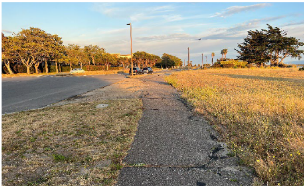
Figure 3 - Older distressed AC pathway and missing curb and gutter
