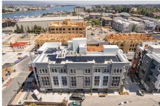
Construction of Bay 37, which will include 39 units offered to very low-, low- and moderate-income households over three phases
