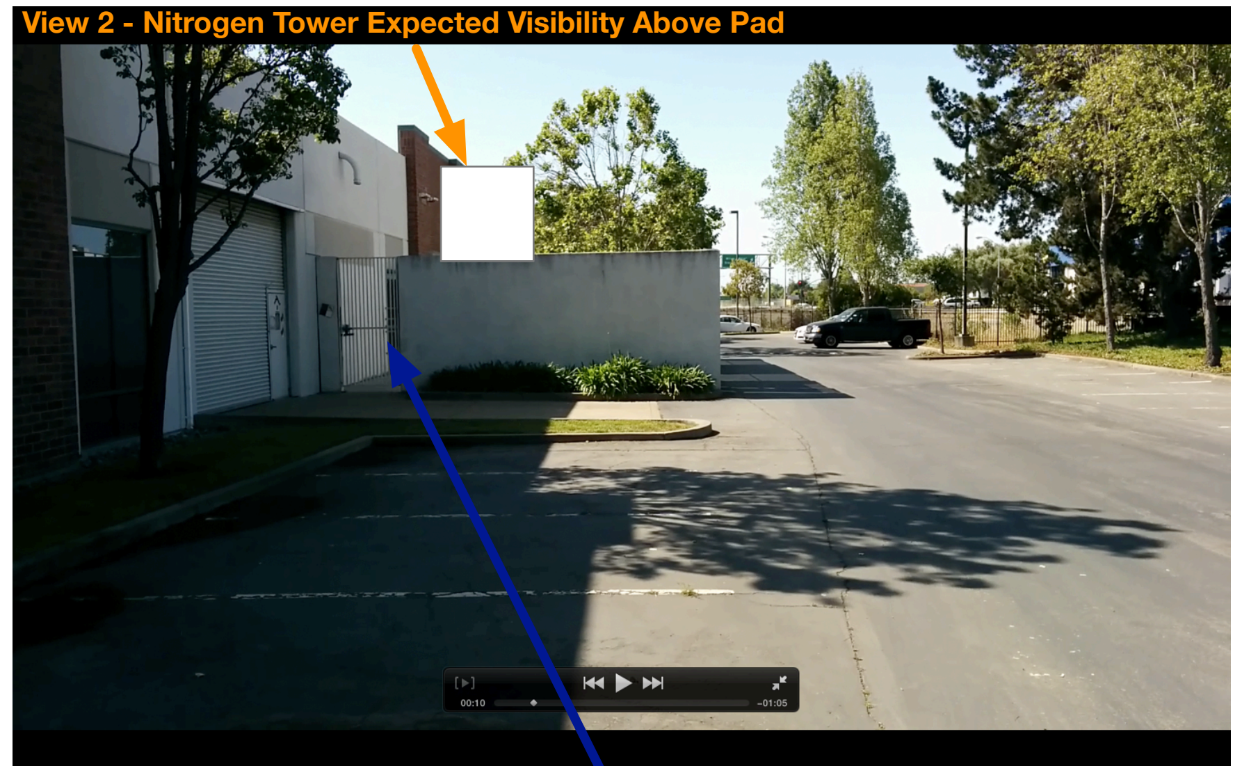
Walls expected to be improved, non-cinder block sections replaced with cinder block Doors may be replaced with solid steel doors. One additional door may be added.
