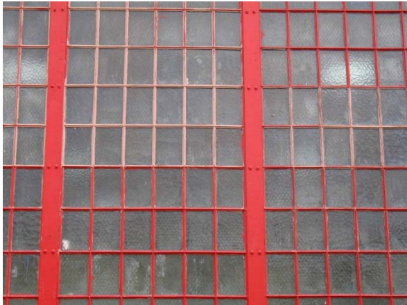
Window with closely spaced muntins and translucent glass, historic industrial building, Alameda Point.
