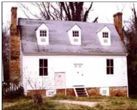
Regrading has protected this masonry foundation wall from excessive damp during its 10-year mothballing. Note the attic and basement vents, temporary stairs, and interpretive sign. Photo: NPS files.
