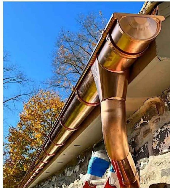
Copper gutters /downspouts
