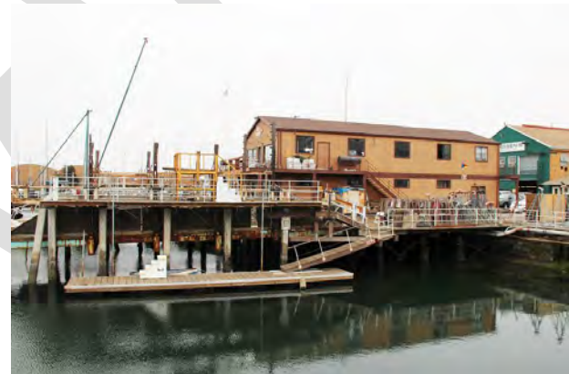
Figure 12. Typical pier, float, and wharf condition, 2016.
