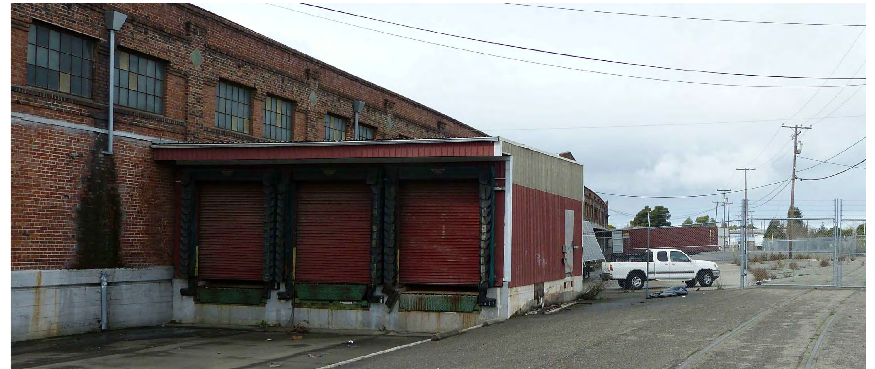
VIEW 2 - EXISTING CONDITION VIEW FROM ENTRANCE RD AND CLEMENT ALONG BUILDING FACADE
