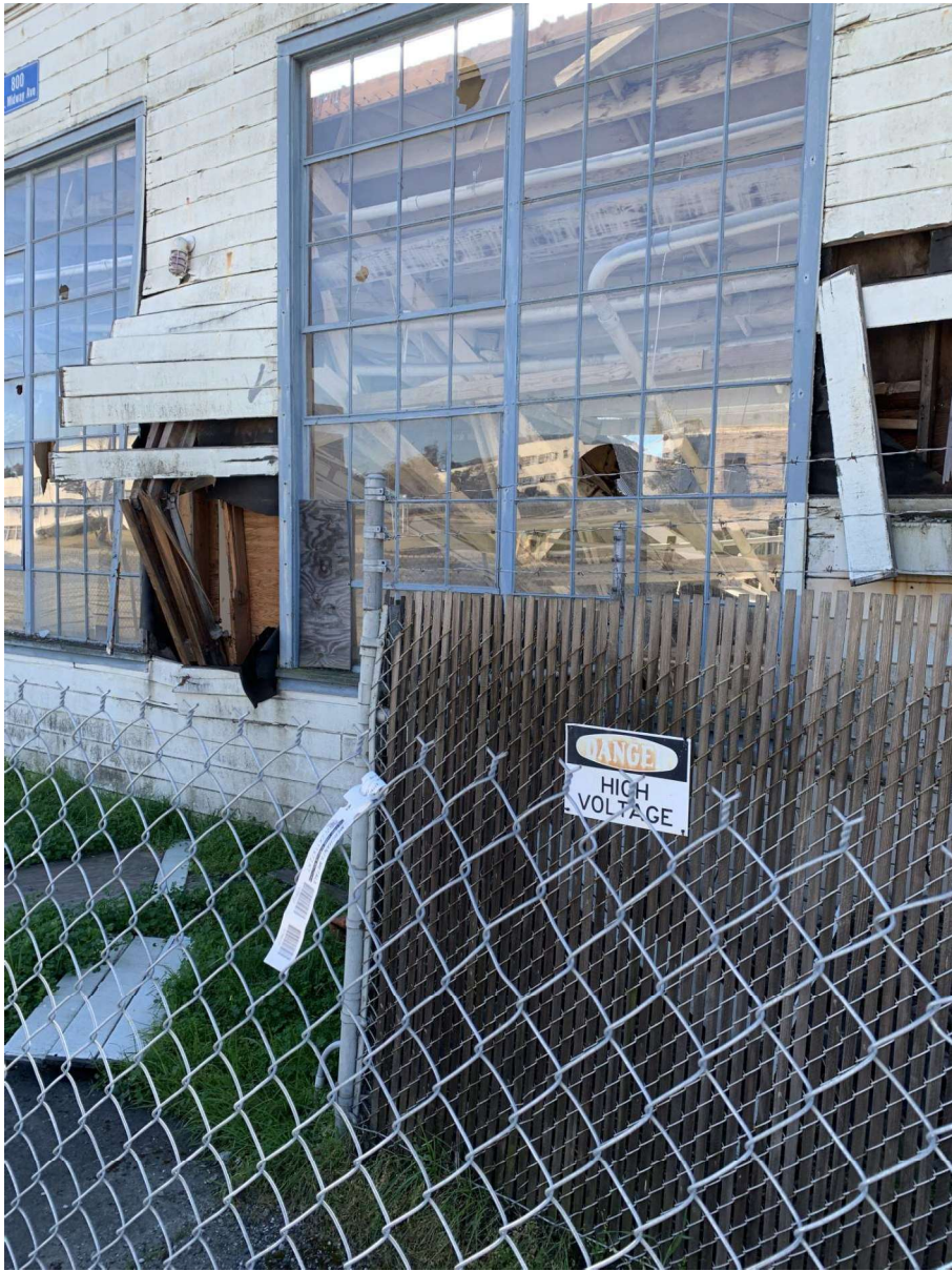
Figure A.4 - Collapsed roof at East side of building.
