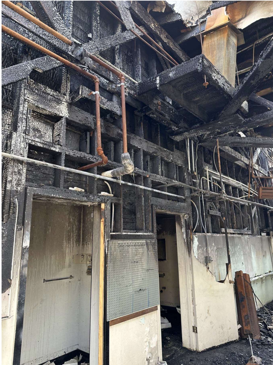
Figure A.6 - Fire damaged wall framing at East end of South wing.
