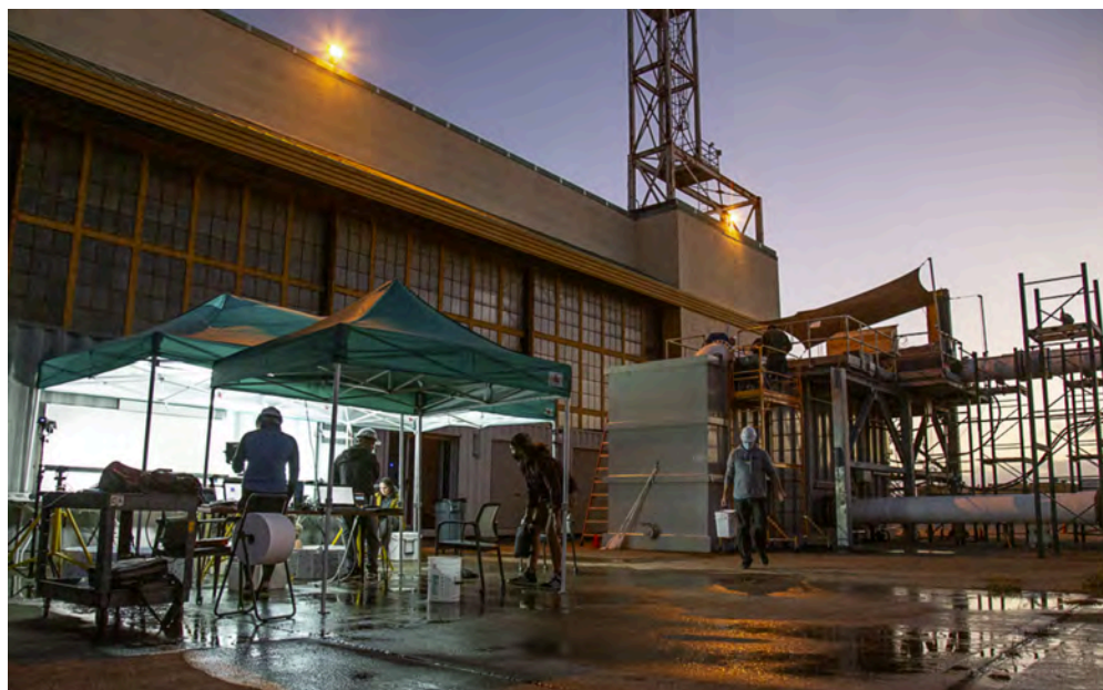
Figure 17: an example of work outside at dusk, showing the security lighting at the top of the building as well as some local lighting used for testing. Temporary rain shelters for test equipment and staff are also shown.
