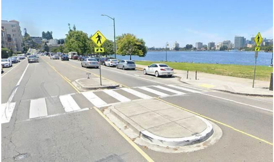
Figure 17: Median Refuge Island at the Intersection of Lakeshore Avenue and Cleveland Cascade in Oakland.
