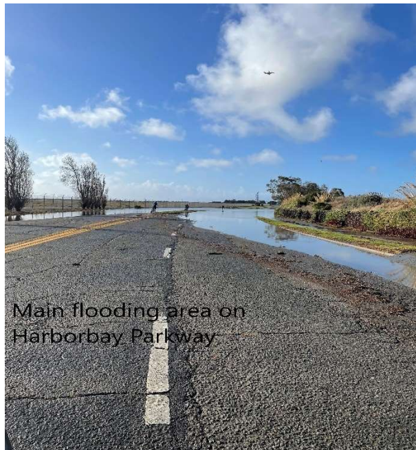
Figure 6 – December 2021 Flooding of Harbor Bay Parkway 1,500 feet North of Maitland Drive
