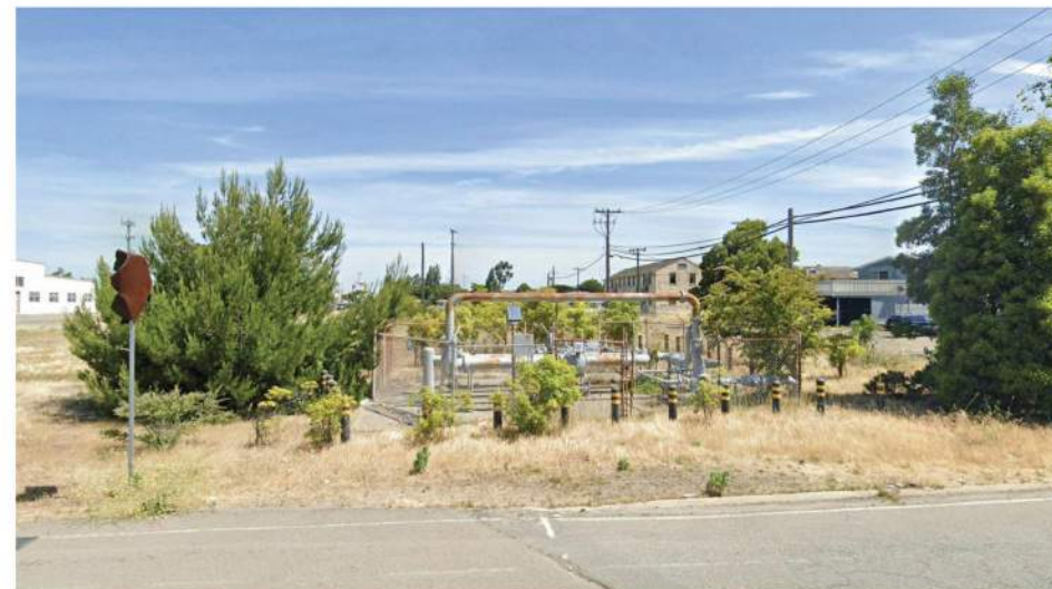
2. PG&E GAS FACILITY
