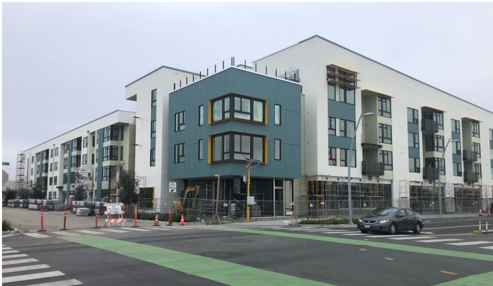
In 2020, work continued on the new housing and the entrance to Alameda Point.
