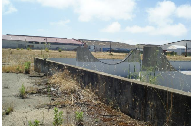
Figure 11. Concrete tank mounts within the enclosure, facing southeast.
