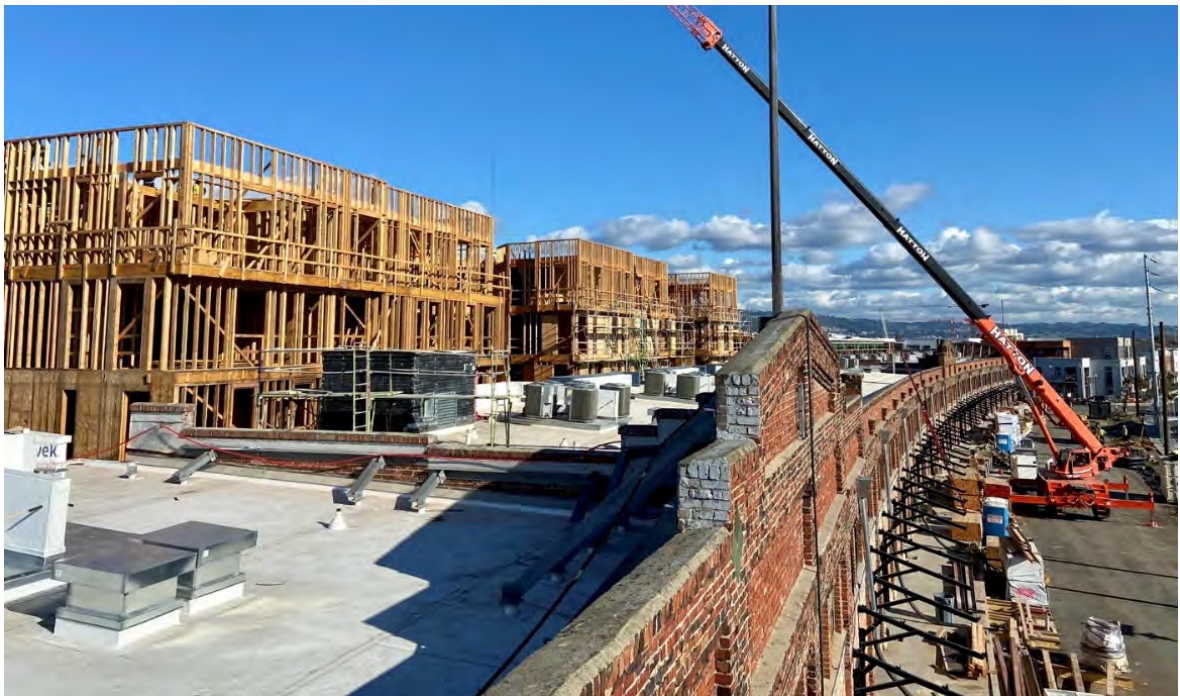
The adaptive reuse and expansion of the historic Del Monte Warehouse will provide for 360 multifamily rental units. Residents will begin moving in in 2022.
