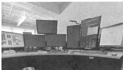
Marin County Fire Dispatch Phase 1
