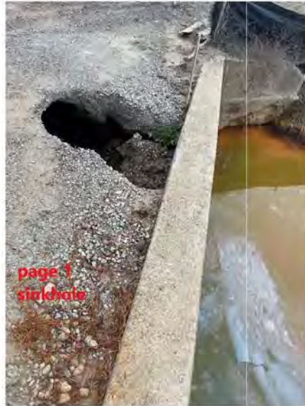
Figure 22 – Sinkhole in 36" PVC Culvert Just Upstream of the Golf Course SDPS Retention Pond on the East Slough
