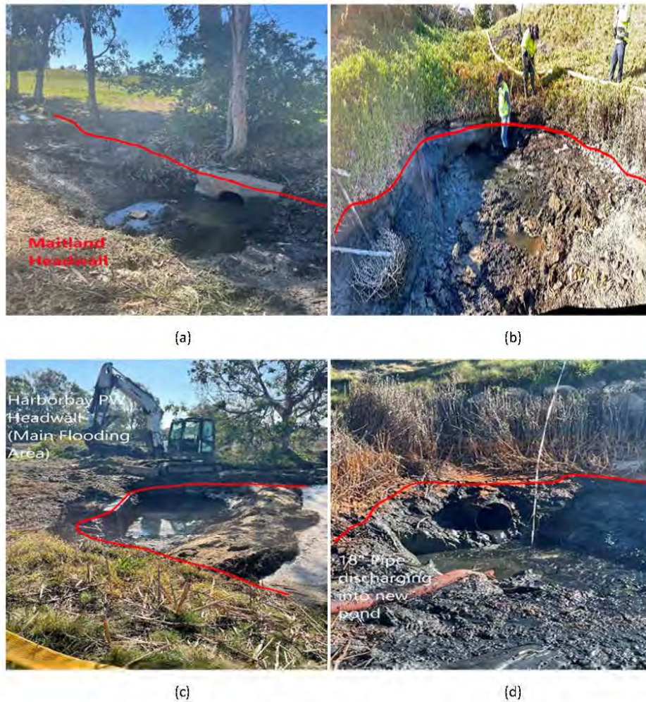
Figure 20 – Images of Storm Sewer Outfalls Blocked with Sediment (Red Line Shows Approximate Level of Sediment Prior to Excavation)
