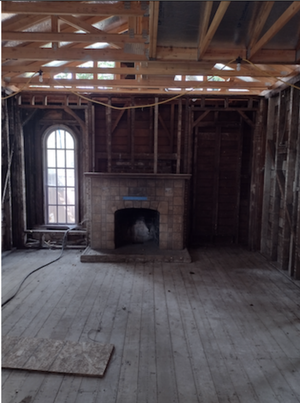
Figure 8. Interior living room fireplace with decorated mantle (GA, October 2025). Note: New trusses possibly show where 2 nd story was removed.
