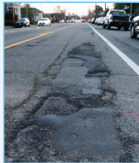
Potholes along Fernside Boulevard that need to be filled
