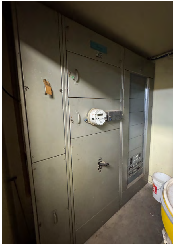
IMAGE A - EXISTING MAIN SWITCHBOARD
