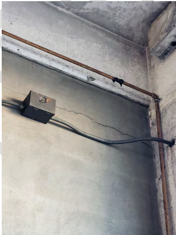
Photo 14: Crack at Interior Infill Wall
