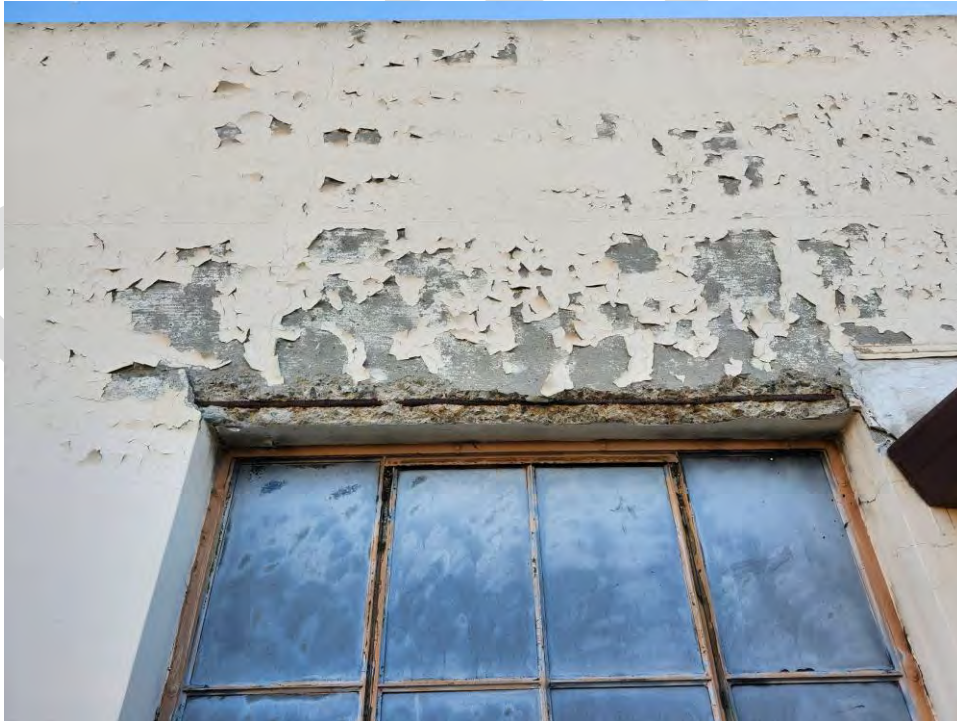
Photo 20: Exposed Reinforcement at Penthouse Gym Window
