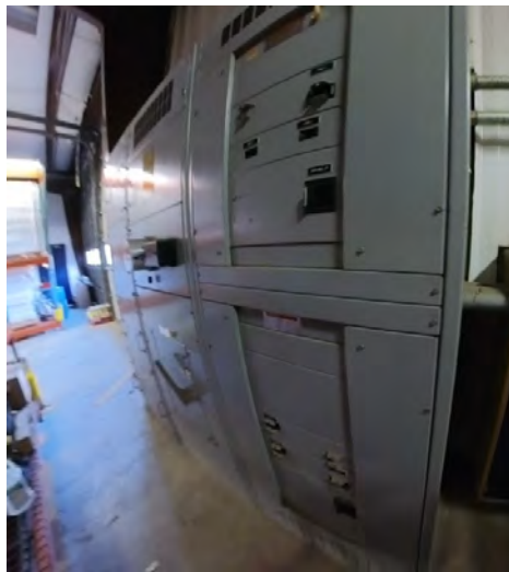
IMAGE A - EXISTING MAIN SWITCHBOARD
