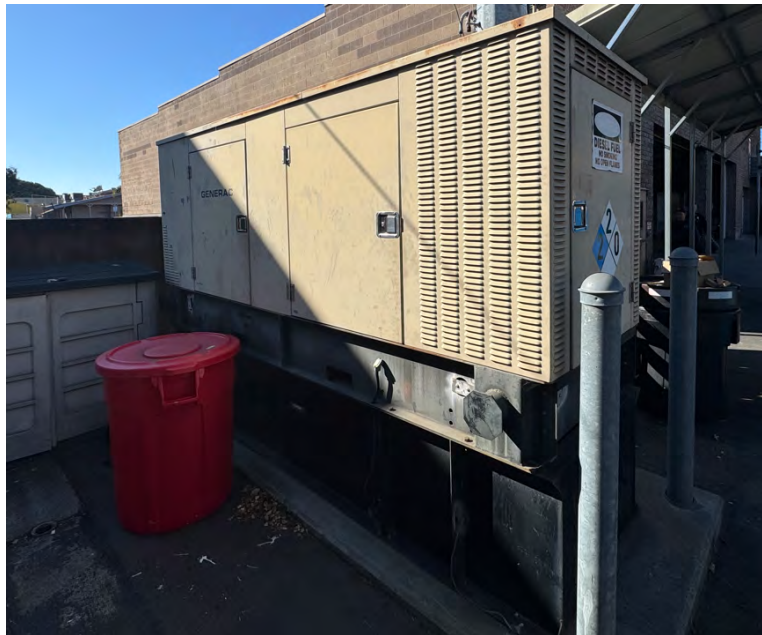
IMAGE B - EXISTING GENERATOR
