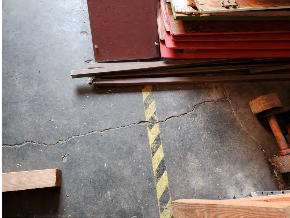
Photo 17: Crack at Second ??? Floor Slab
