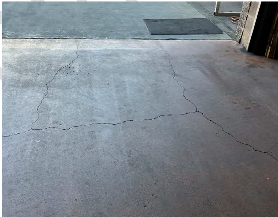
Photo 10: Cracking in Main Apparatus Bay Slab
