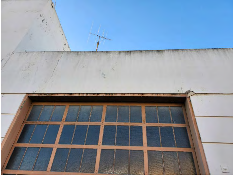
Photo 9: Exterior Cracks at Northern Face
