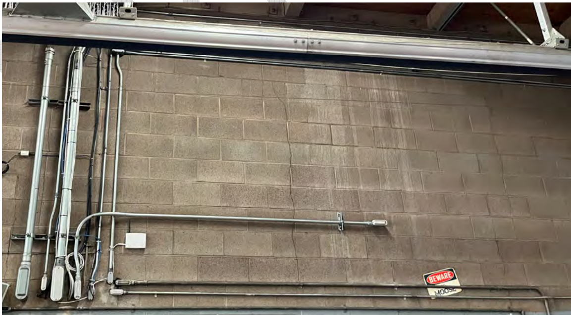
Photo 8: Interior of Apparatus Bay – Cracks in CMU Wall
