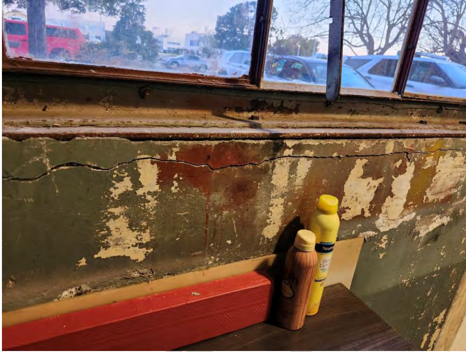
Photo 15: Crack at Classroom Window Concrete Wall
