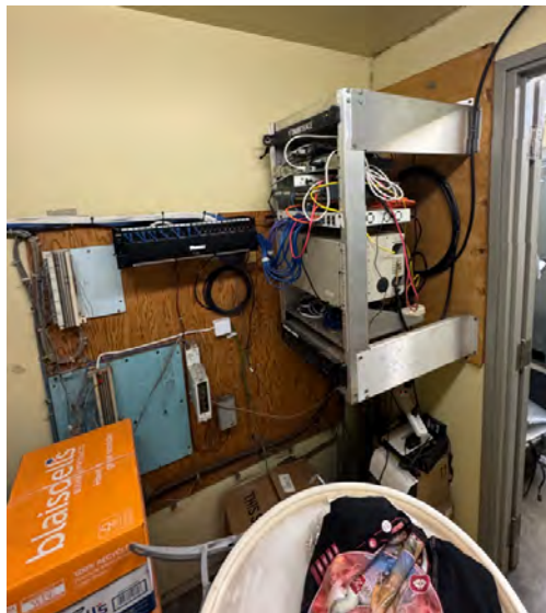
IMAGE B - TELEPHONE BACKBOARD
