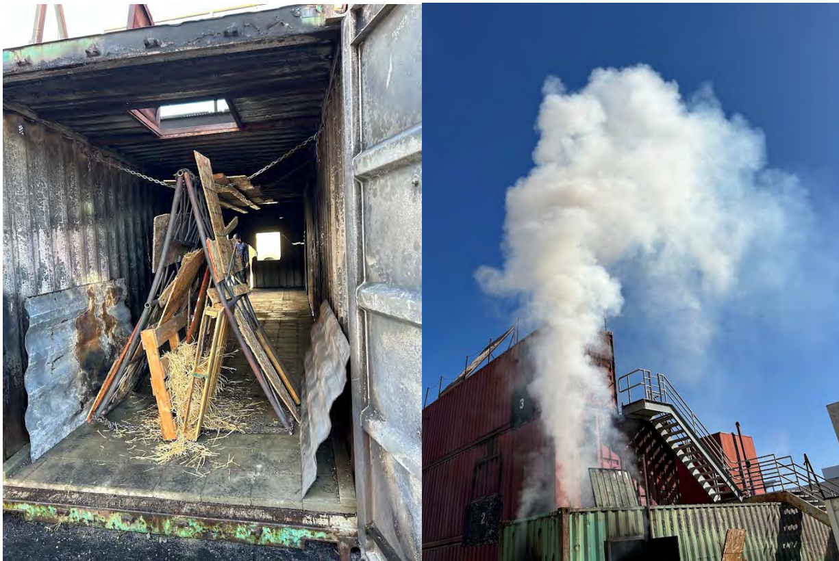
Figure 2. Smoke release through roof vent on storage container. Fan and HEPA filter recommended at this exit point as an engineering control.
