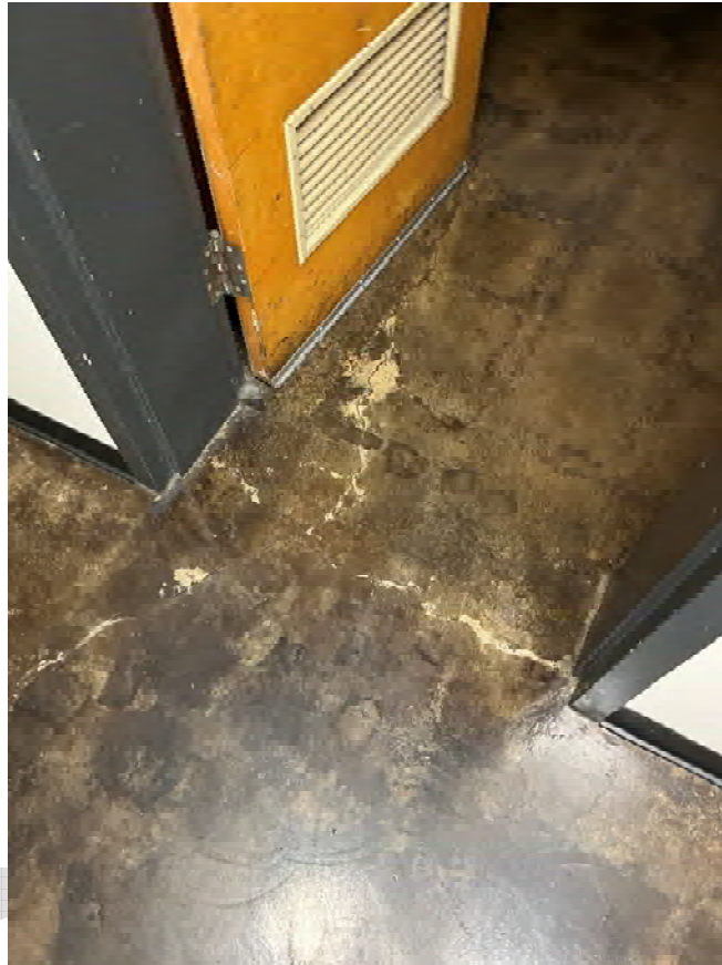
Photo 11: Cracking in Main Apparatus Bay Slab
