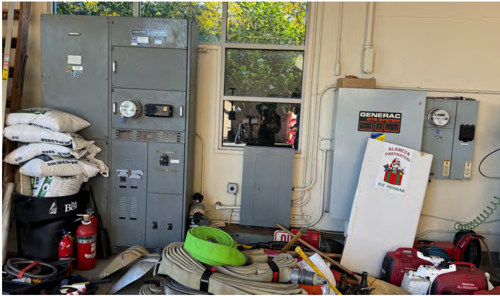
IMAGE A - EXISTING MAIN SWITCHBOARD
