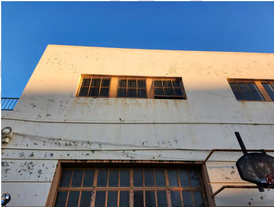
Photo 8: Exterior Cracks at Southern Face Two Story
