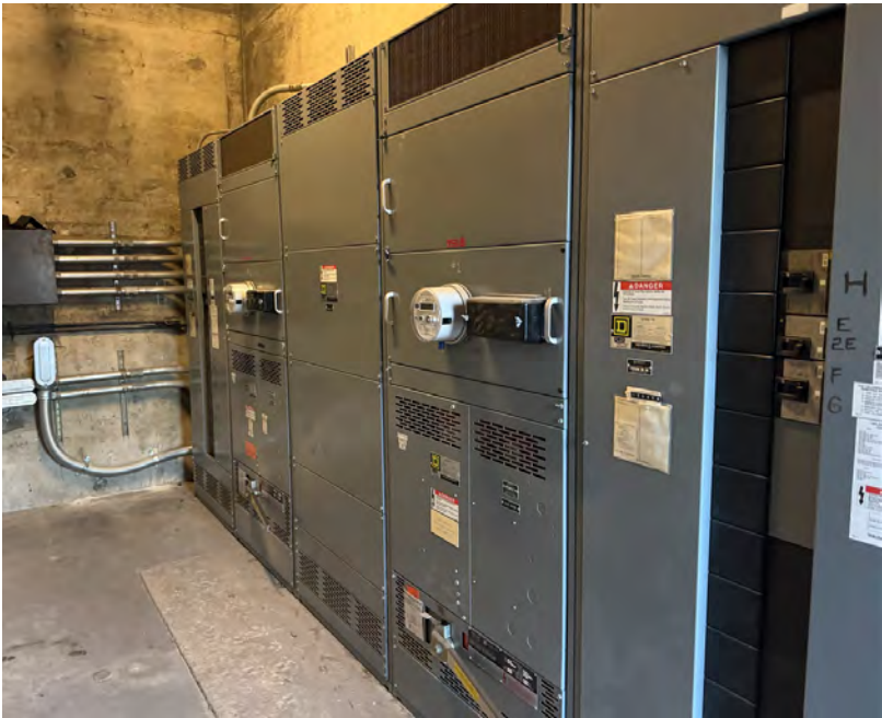
IMAGE A - EXISTING MAIN SWITCHBOARD
