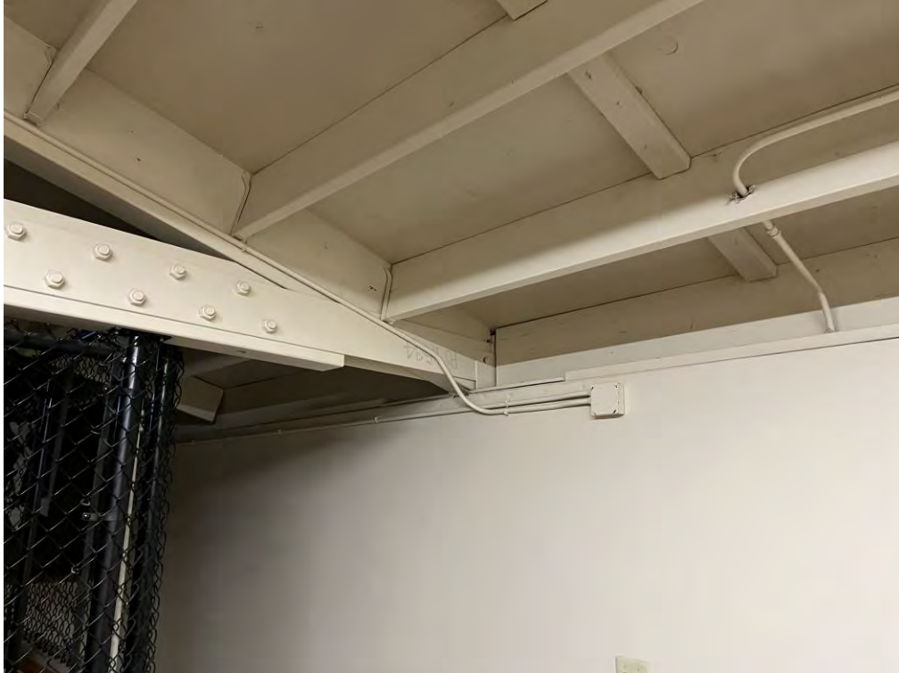
Photo 5: Apparatus Bay – Truss to Wall Connection
