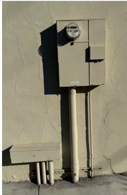
IMAGE A - EXISTING METER/MAIN SERVICE
