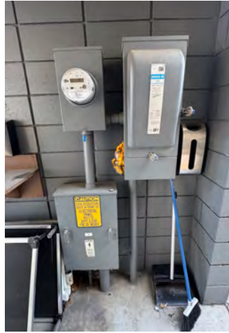
IMAGE A - EXISTING METER SERVICE AND SERVICE DISCONNECT
