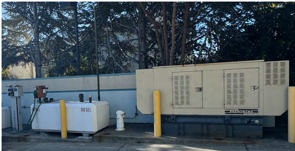
IMAGE B - EXISTING GENERATOR
