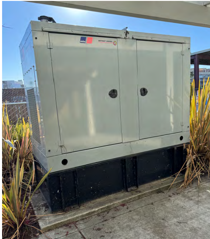
IMAGE D – EXISTING GENERATOR
