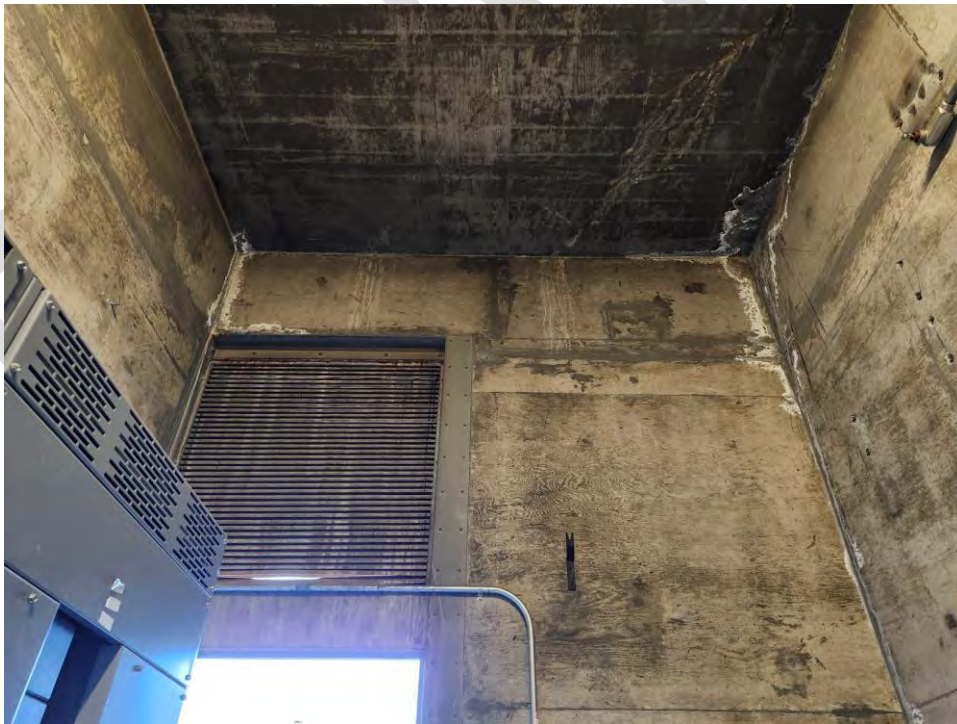
Photo 12: Water Intrusion at Mechanical Room Concrete Roof Slab and Wall
