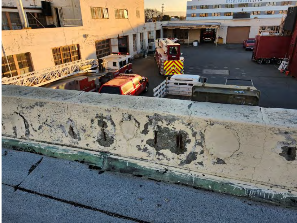
Photo 21: Exterior Damage – Exposed Reinforcement at Roof Parapet Concrete
