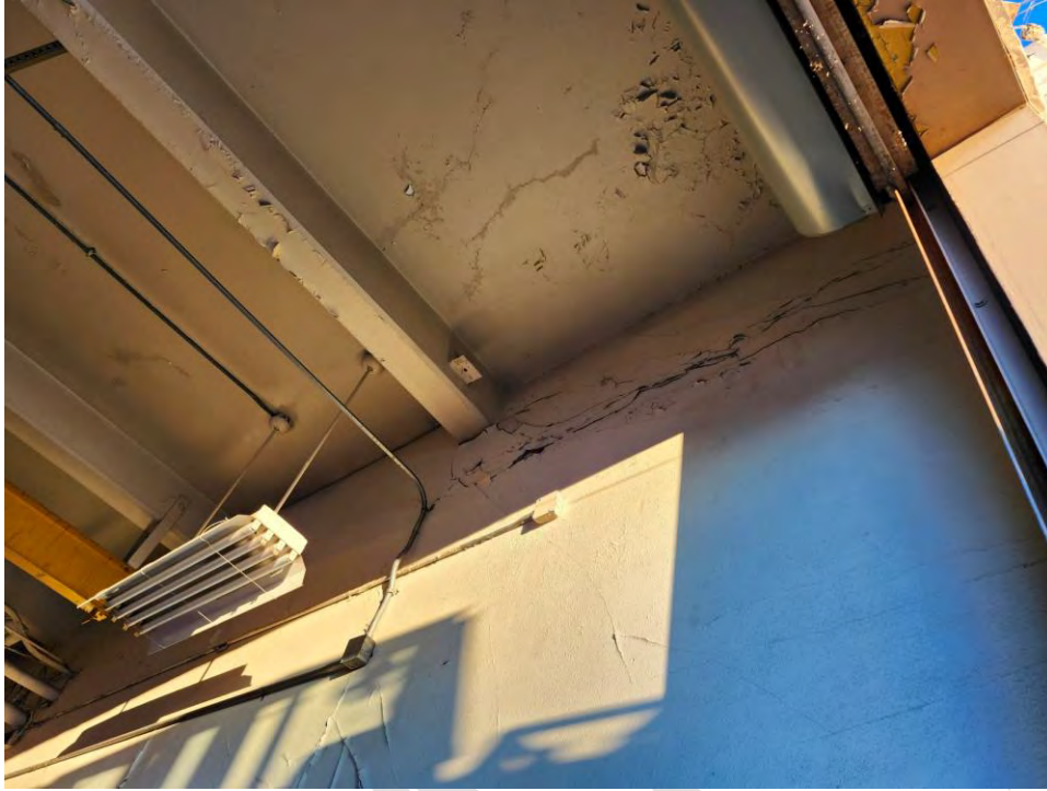
Photo 13: Cracks at Apparatus Bay Wall and Ceiling
