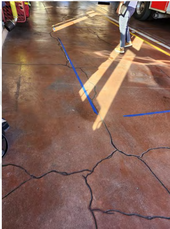
Photo 10: Cracking in Main Apparatus Bay Slab
