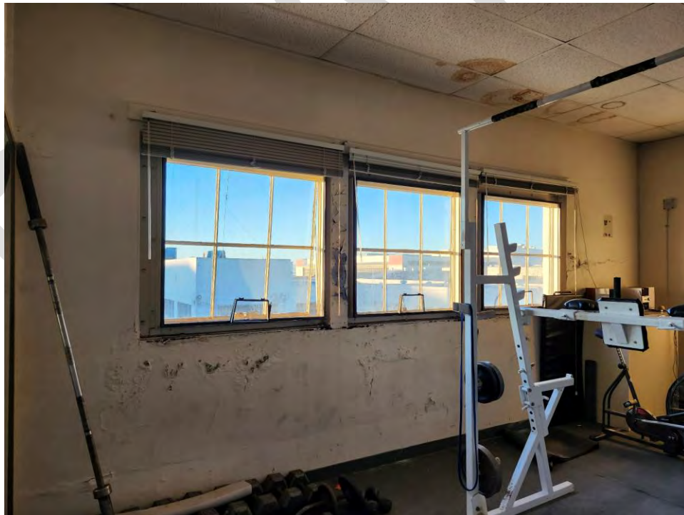
Photo 22: Cracks at Exterior Wall of Penthouse Gym
