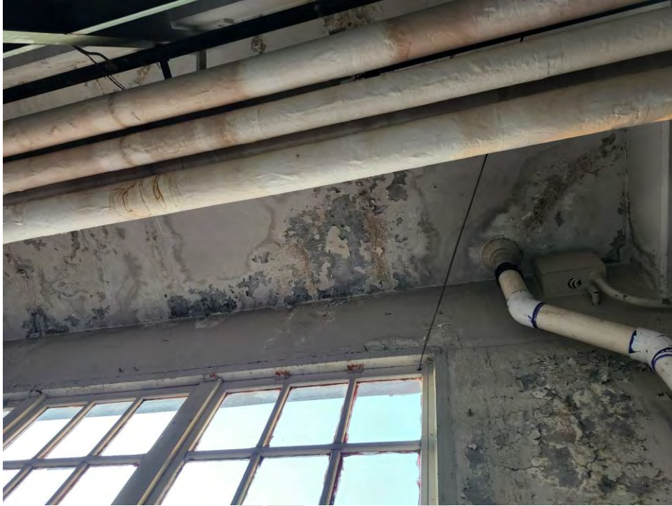
Photo 11: Water Damage at Concrete Roof Slab
