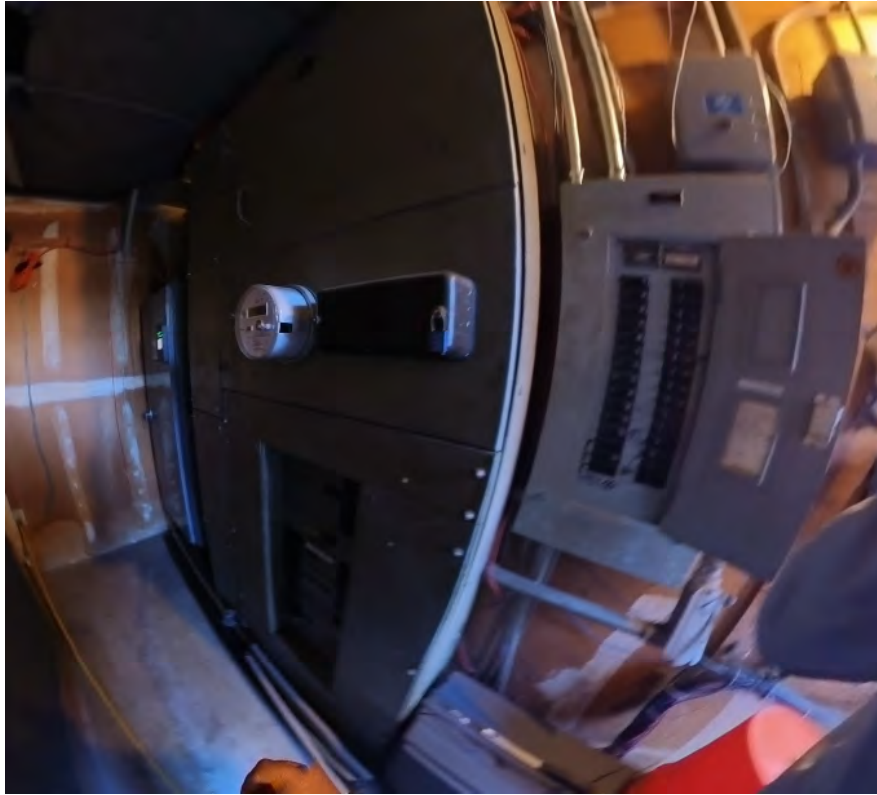
IMAGE A - EXISTING MAIN SWITCHBOARD
