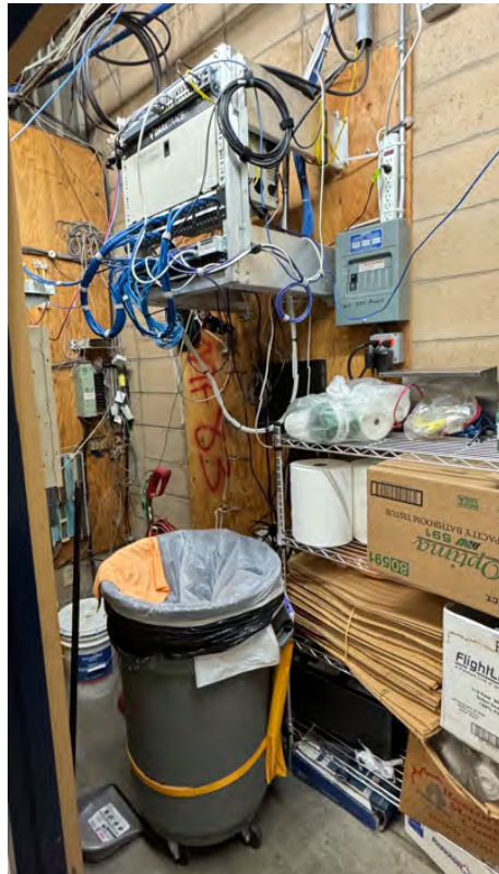
IMAGE B – TELEPHONE BACKBOARD
