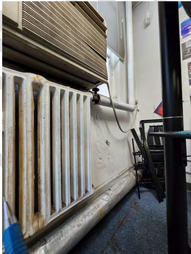
Photo 18: Interior Water Damage at Conference Room
