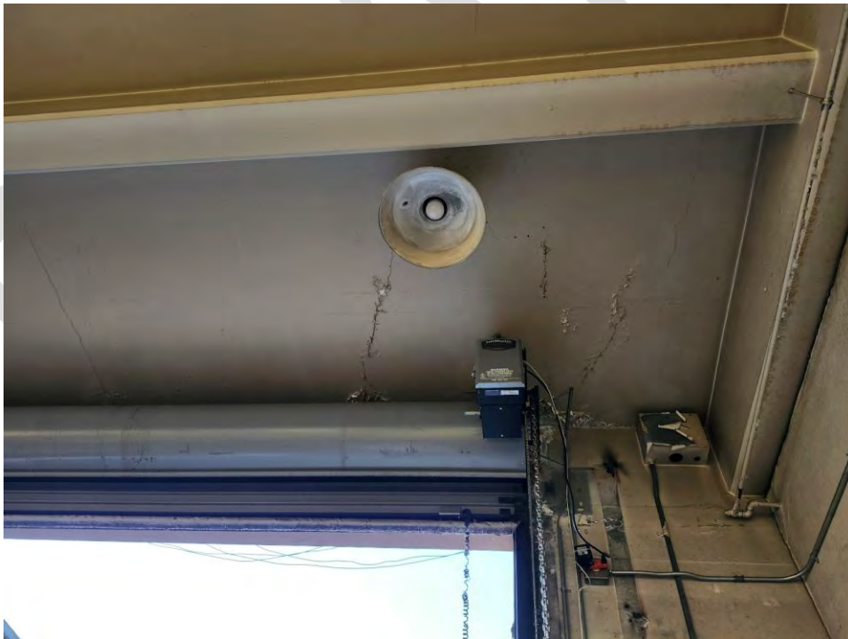
Photo 10: Roof Slab Cracks at Apparatus Door
