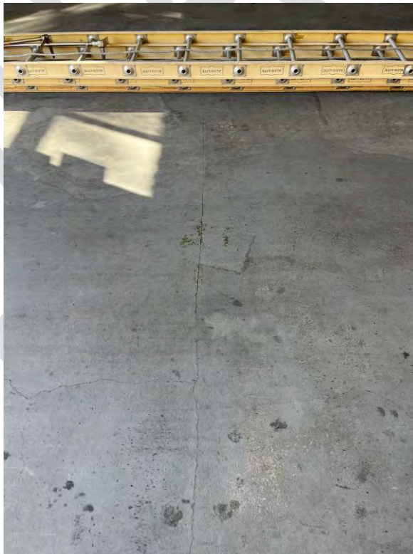
Photo 6: Interior of Apparatus Bay – Cracks in Slab
