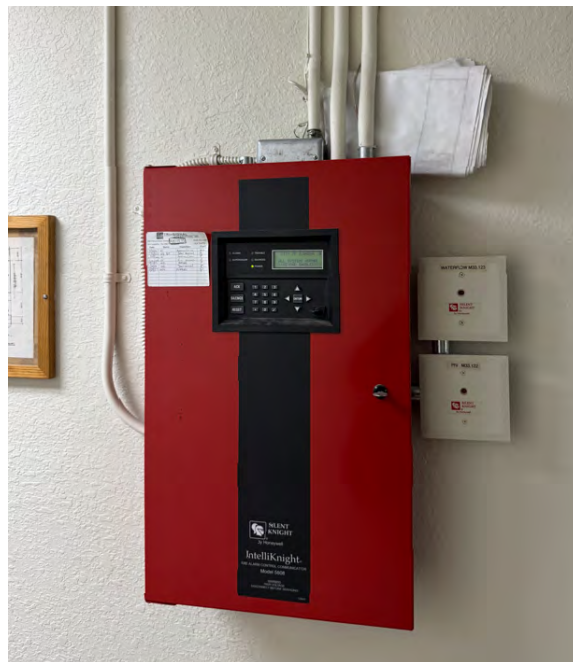
IMAGE C – EXISTING FIRE ALARM
