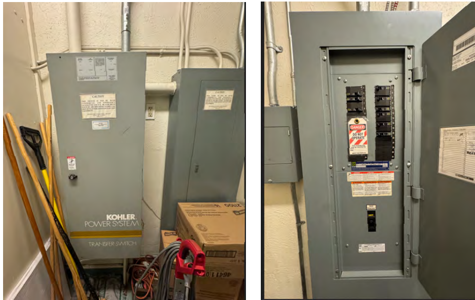
LEFT PICTURE (ATS) AND SERVICE PANEL RIGHT PICTURE SUBPANEL WITH LOAD CENTER IMAGE B - EXISTING PANELS AND ATS
