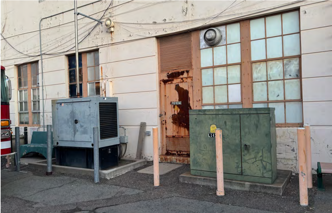
IMAGE B - EXISTING GENERATOR AND UTILITY TRANSFORMER
