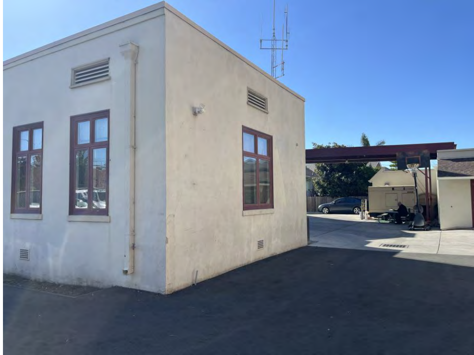
Photo 11: Minor Chipping at Exterior Stucco
