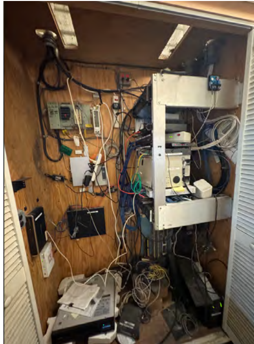
IMAGE E - EXISTING IT CLOSET
