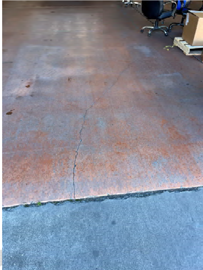
Photo 9: Cracking in Main Apparatus Bay Slab
