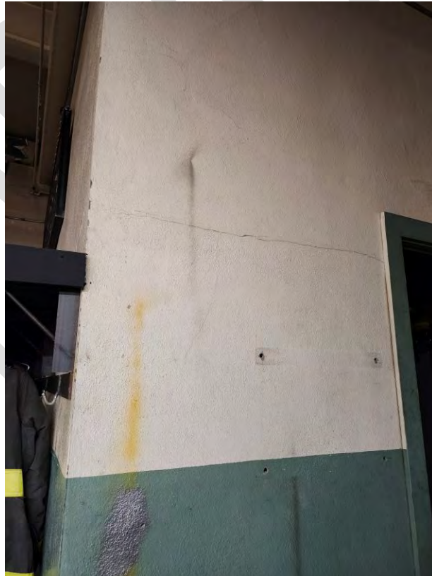
Photo 16: Crack at Locker-room Concrete Wall
